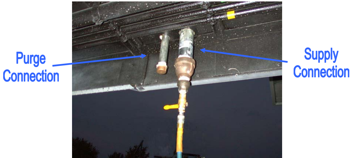
Figure 38: Fire Suppression Supply and purge connections
