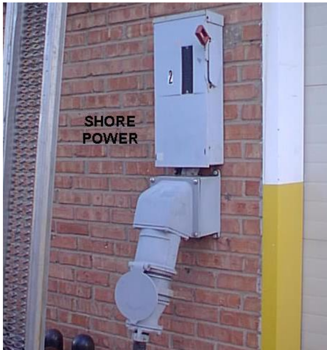
Figure 8: Shore Power Connection.
