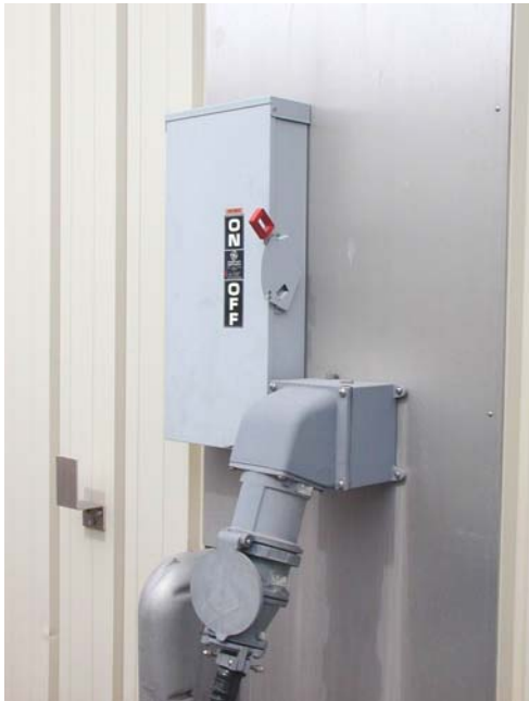
Figure 45: Shore Power Connection
