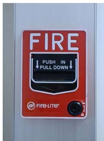
Figure 33: Fire Alarm Pull Station
