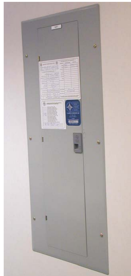
Control Room Panel
