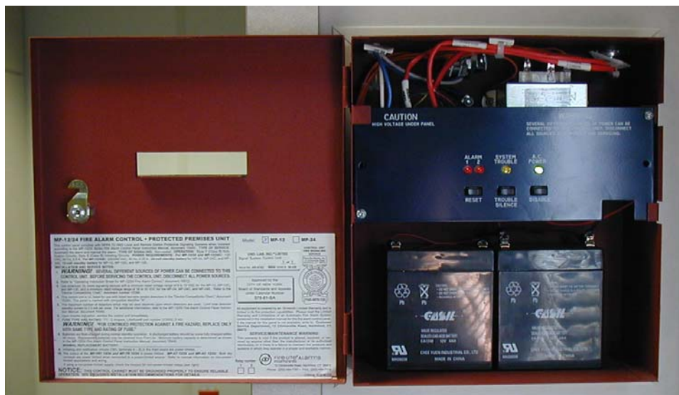
Figure 3: Fire Alarm Control Panel
