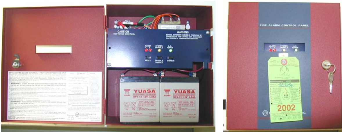
Figure 32: Fire Alarm Control Panel
