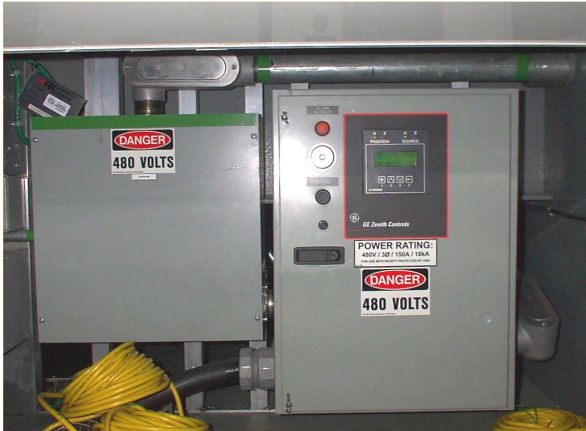
Figure 24: ATS Control Panel
