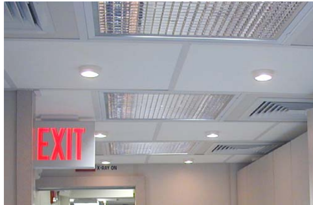
Figure 65: Control Room Lighting
