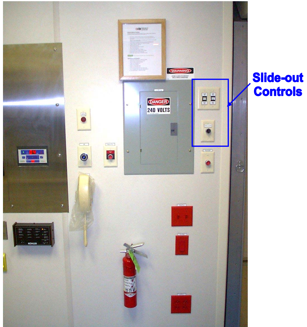
Figure 11: Procedure Room Controls
