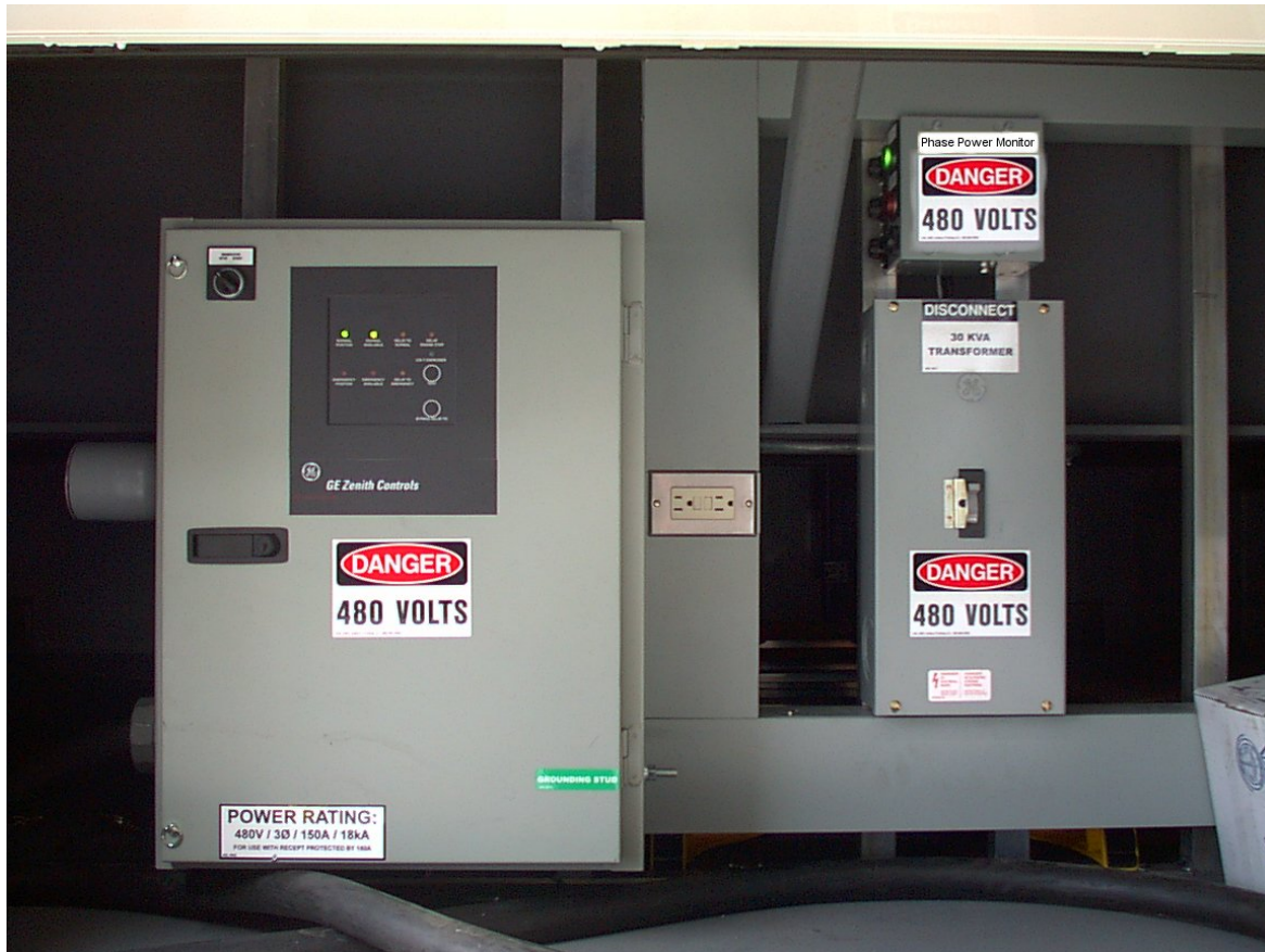
Figure 47: 480V AC ATS and Phase Power Monitor
