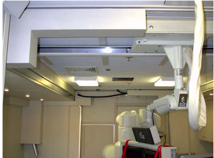
Figure 66: Procedure Room Lighting
