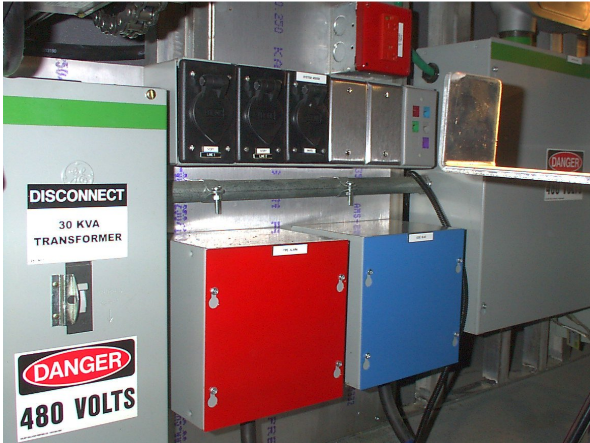
Figure 37: Fire Alarm and Code Blue Alarm Junction Boxes
