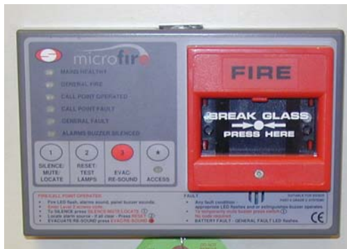
Fire Alarm Pull Station and Fire Detection System Control Panel
