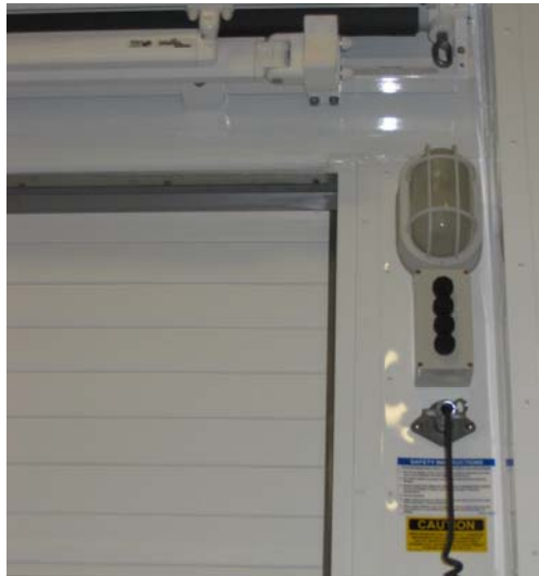
Figure 45: Staff Door Lighting
