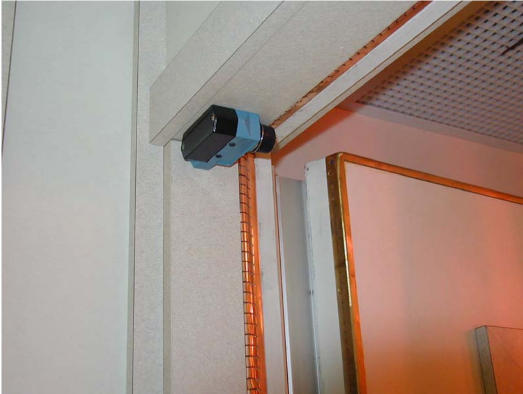
Close up of RF door trim
