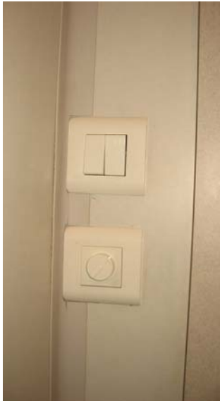
Control Room, and Equipment Room Lighting
