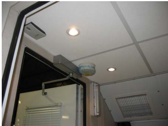
Figure 46: Equipment Room Lighting
