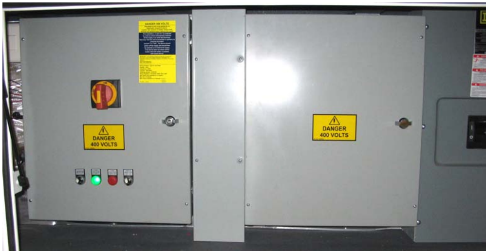
Figure 27: 400/230V AC Electrical Panel Controls
