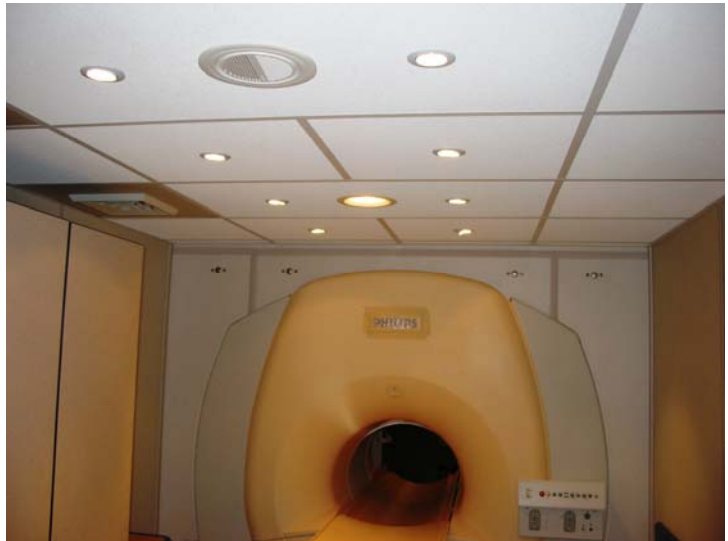
Figure 48: Scan Room Lighting
