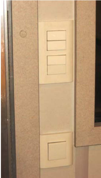
Scan Room Lighting
