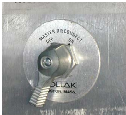
Figure 37: Hydraulic Lift Master Disconnect Switch
