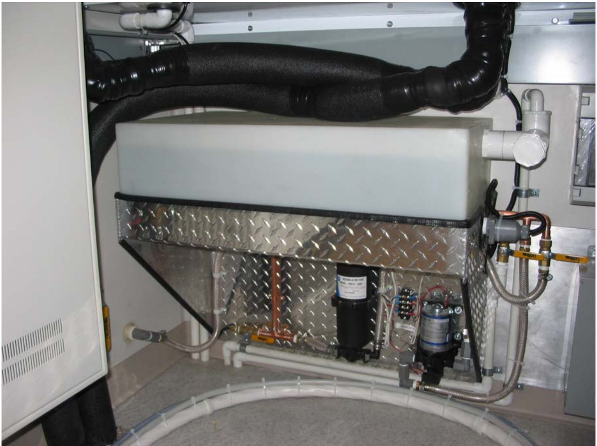
Figure 29: Humidifier Supply Tank
