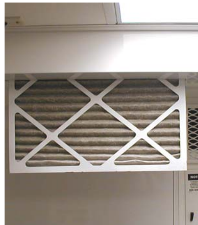
HVAC Filter Access
