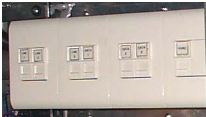
Figure 22: Phone & Data Line Connections
