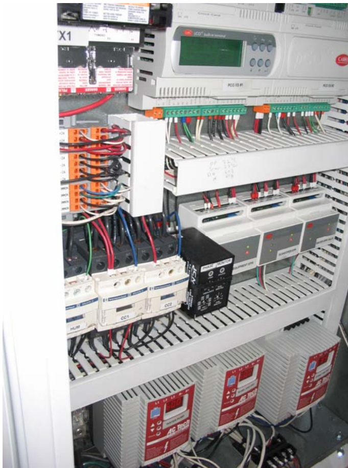
Figure 31: A/C / Chiller Control Panel
