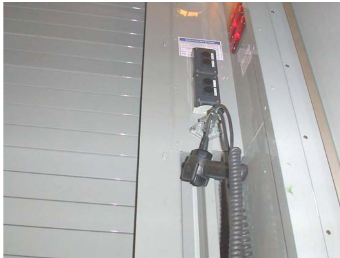
Figure 38: Hydraulic Lift Controls
