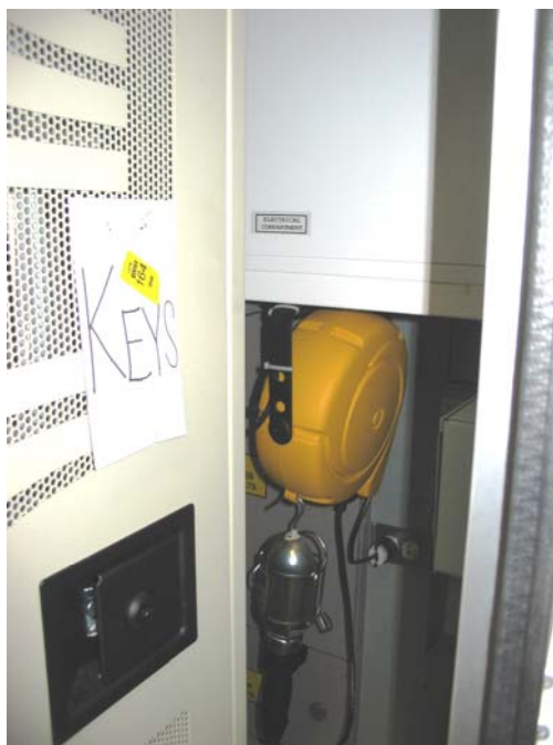
Figure 14: Equipment Room Overall
