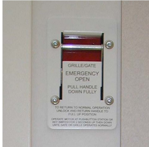
Figure 8: Roll Door Emergency Release
