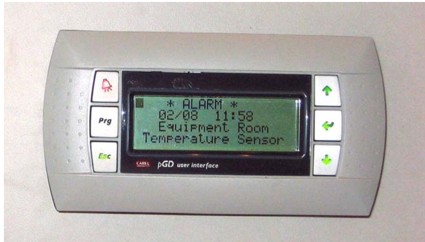
Figure 32: PGD Alarm Panel
