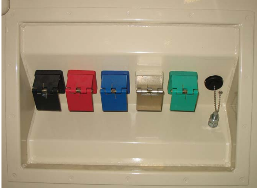
Figure 25: Generator Power Cable to Trailer Cam-lock Connectors
