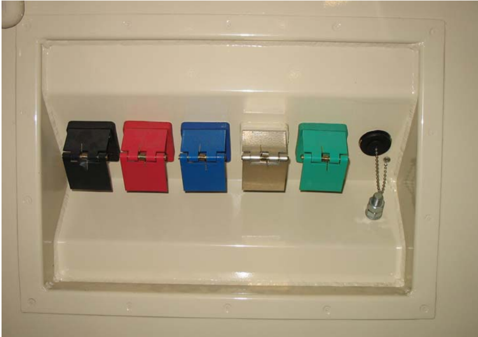
Figure 14: Generator Cam-lock Connectors
