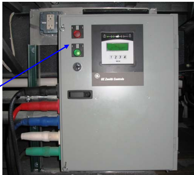
Figure 29: 220V AC Phase Power Monitor
