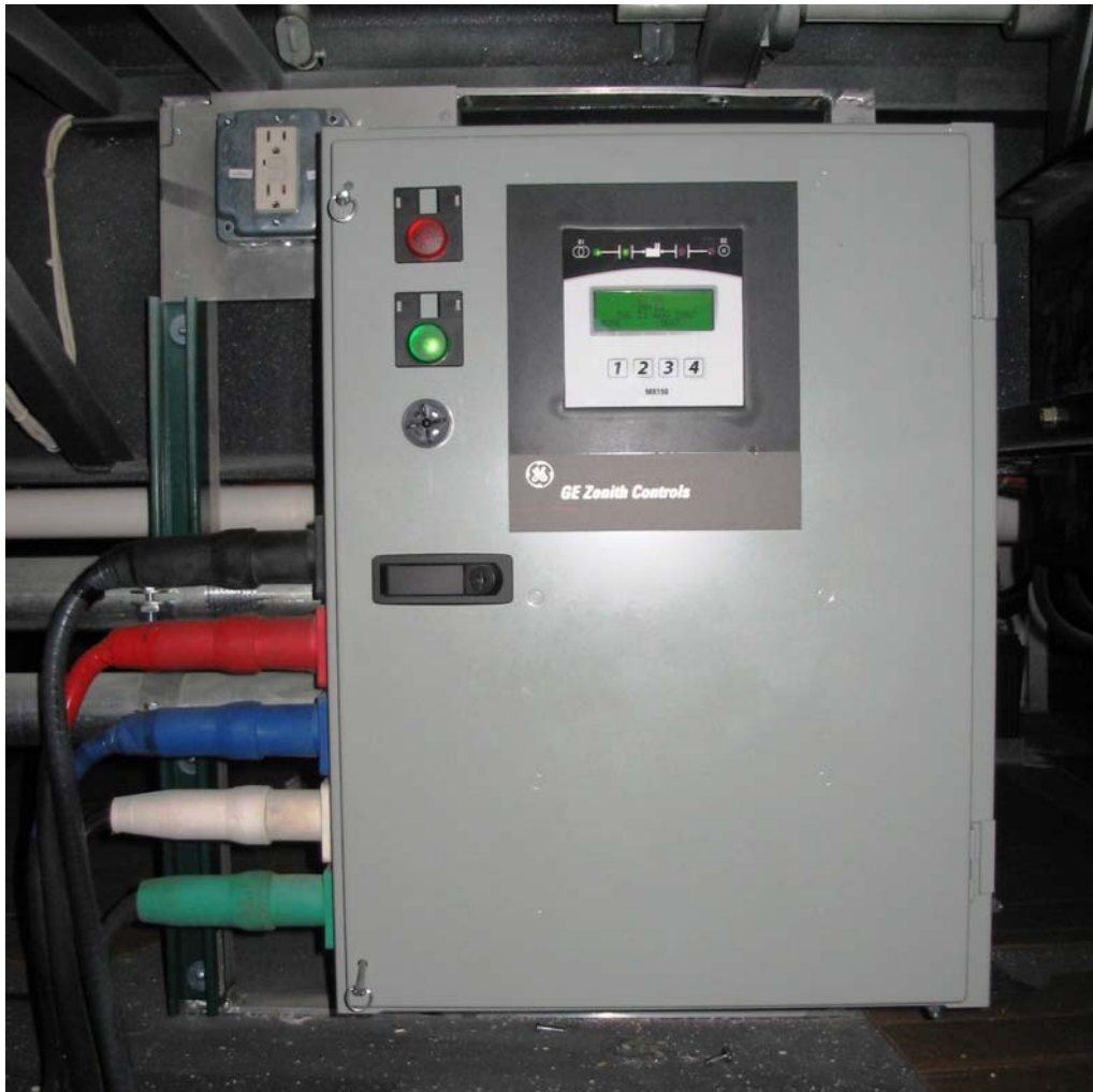
Figure 10: Automatic Transfer Switch (ATS)
