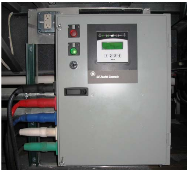
Trailer Underbody Power Connections
