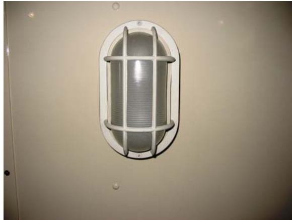
Figure 40: Entry Door Lighting
