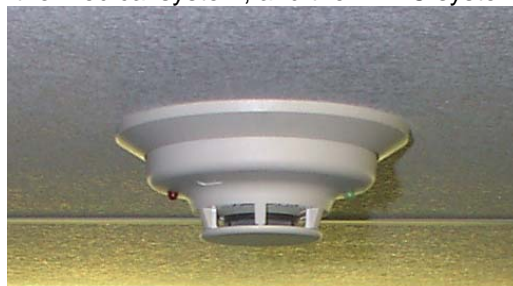
Figure 4: Smoke / Carbon Monoxide Detector
