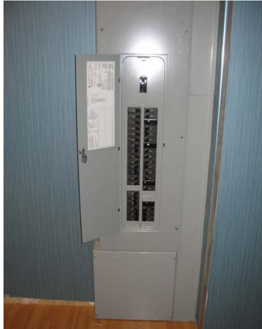
Figure 27: 220/127V AC Electrical Panels
