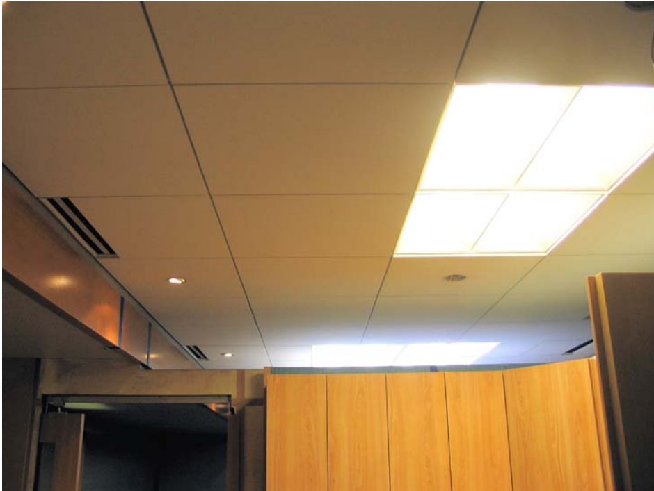
Figure 41: Interior Overall Lighting
